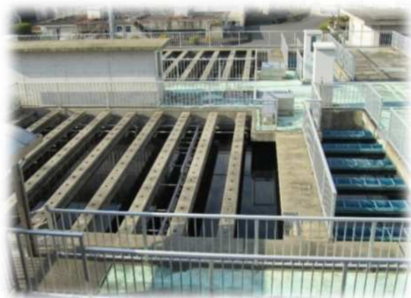
[傾斜板式沈澱池]
